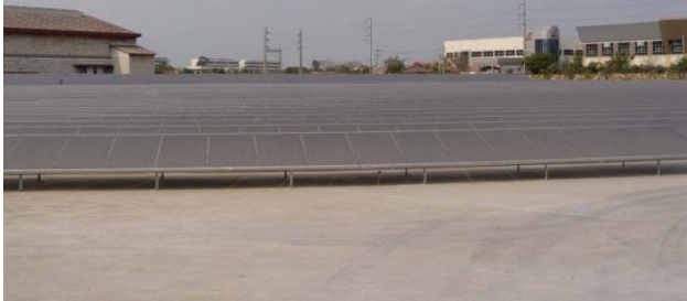
1.3 MW solar farm in Chachoengsao
